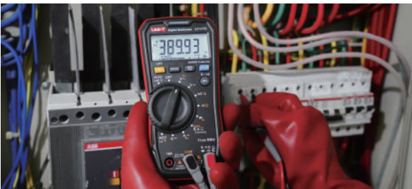
AC voltage measurement
