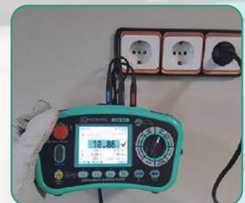
Loop test from a wall socket
